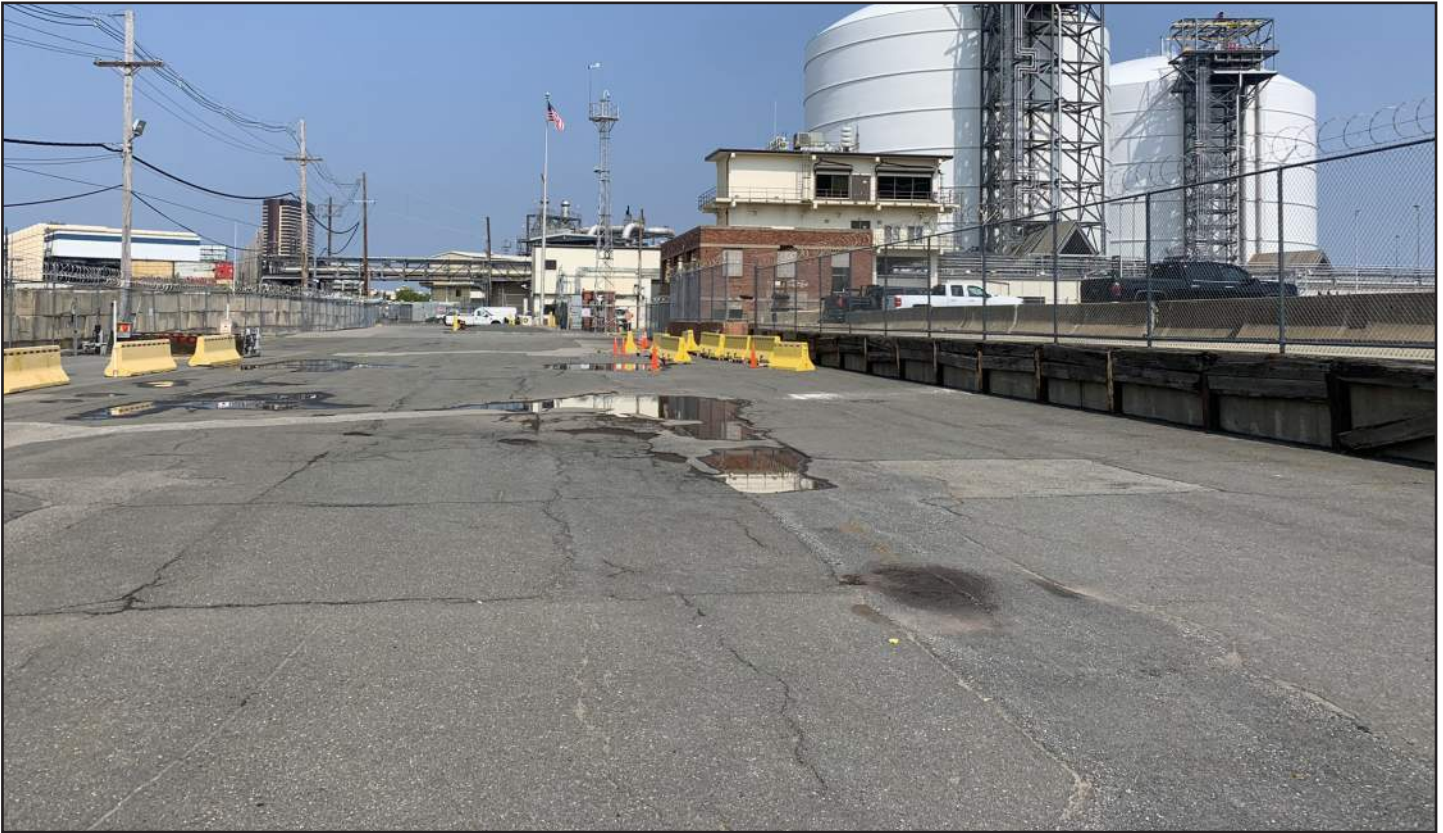
Photograph 17: View looking northwest towards Constellation Energy
