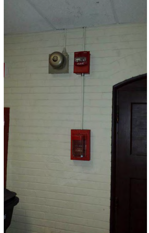
Horn Strobe and Pull Station
