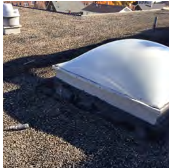
Flashings at skylights, roof fans & equipment deteriorated
