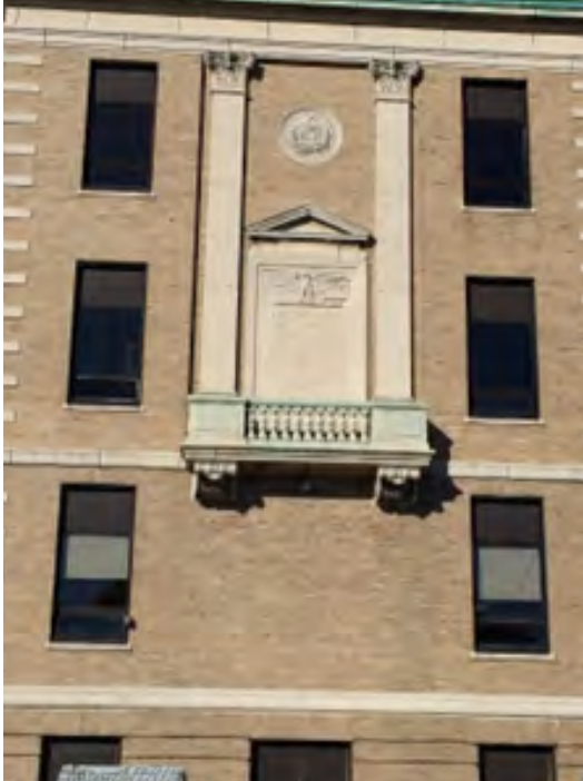
Copper cornice flashings deteriorating
