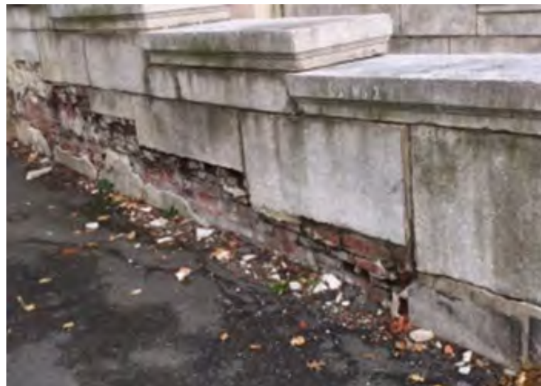
The exterior site walls at the side entrance are severely deteriorated and will require removal and replacement.
