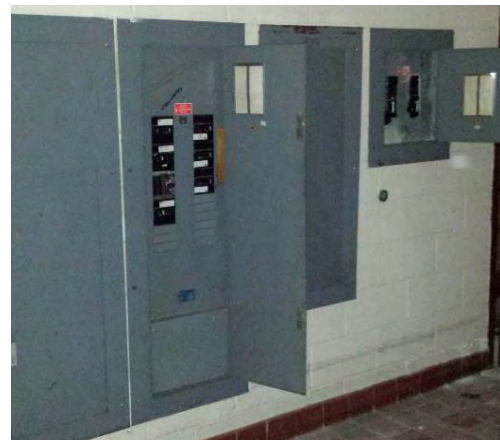
Panelboards in Kitchen
