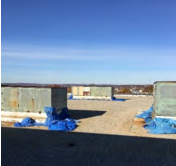
Failed and deteriorating mechanical units
