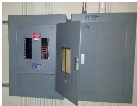
Panelboards in Electrical Room
