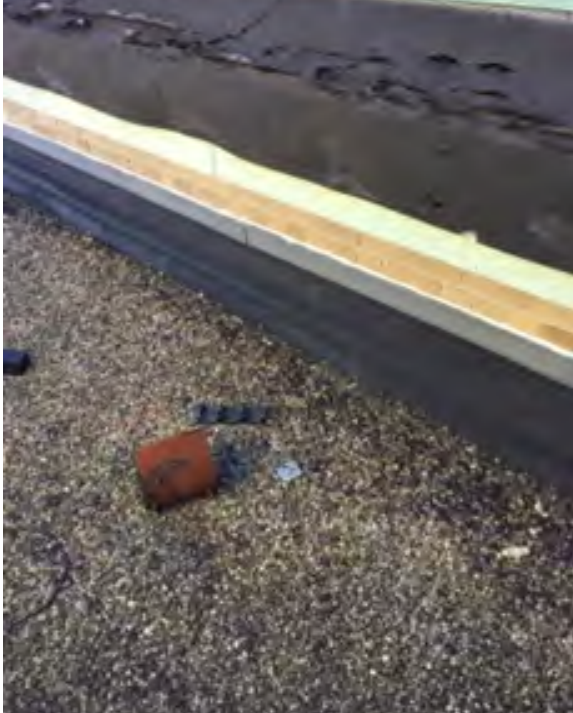
Flashings deteriorated and useless
