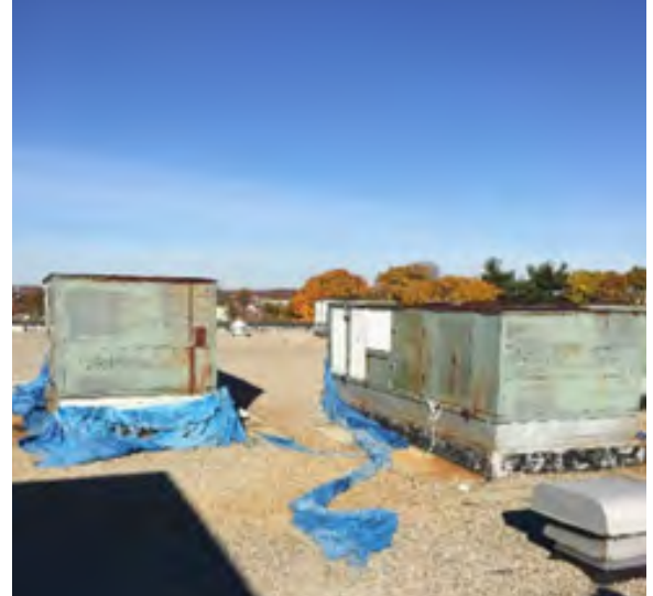
Failed and deteriorating mechanical units
