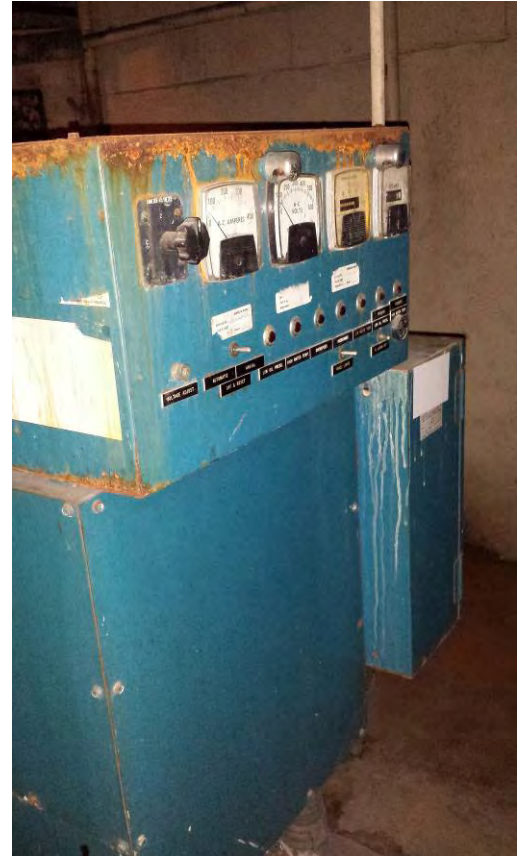
Generator Control Panel
