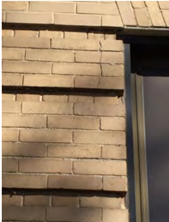
Masonry cracks and re-pointing required
