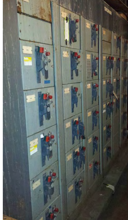
Motor Control Center
