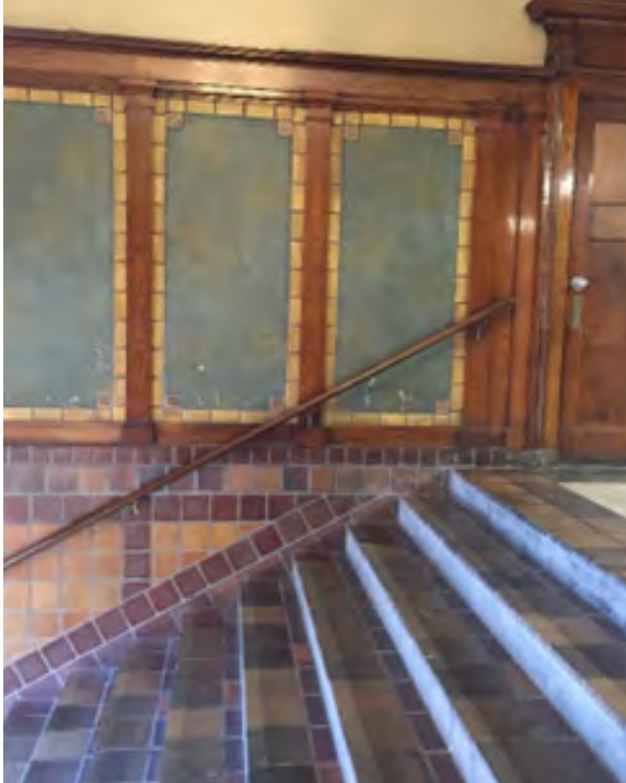
Existing interior main entry stairs non accessible
