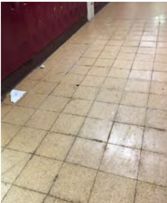
VAT & VCT worn throughout school
