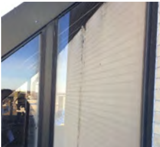
Exterior wall light leaking at inside
