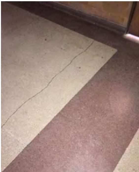
Existing terrazzo floors and cracking
