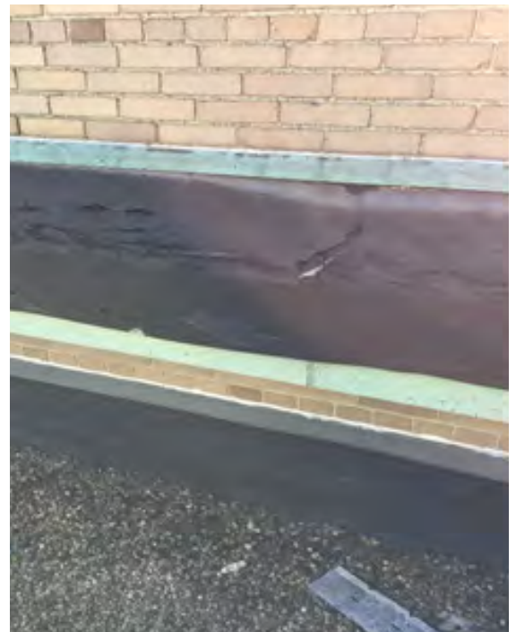
Deteriorated flashings, both copper and membrane
