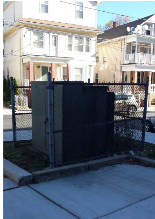
Pad Mounted Utility Transformer
