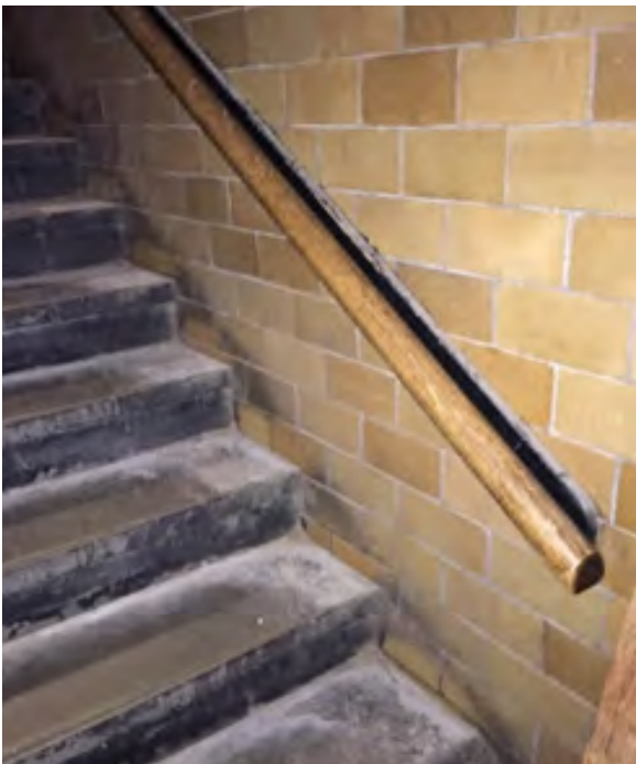
Non-Compliant rails and stair tread nosings
