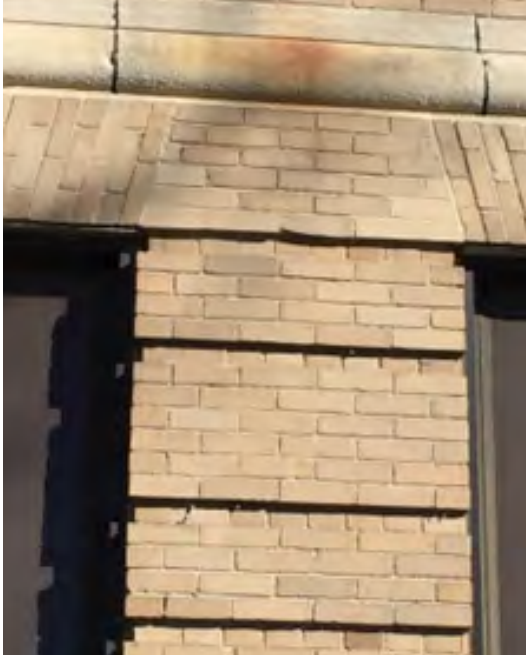
Continuous cast stone bands require repointing
