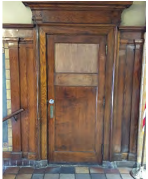
Existing interior door and trims. Hardware non-compliant.
