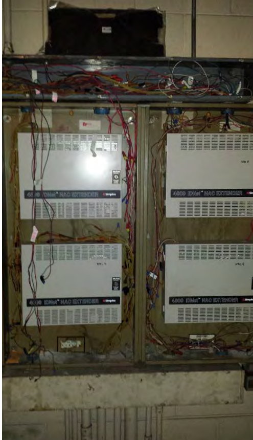
Original Control Panel with new Equipment
