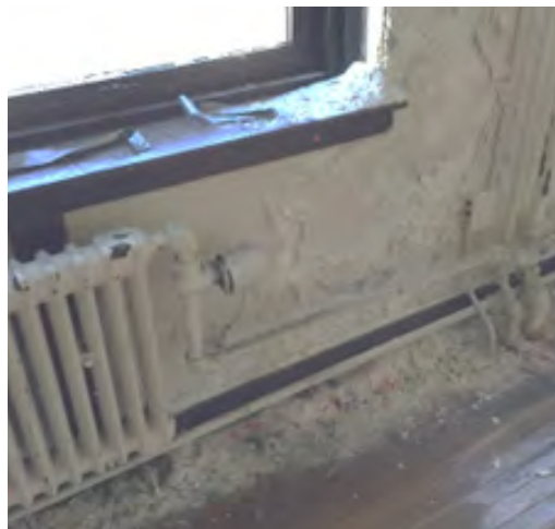
Water migration and damage to interior surfaces
