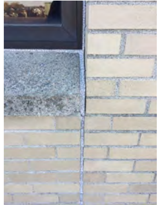
Masonry and window openings require repointing and caulking
