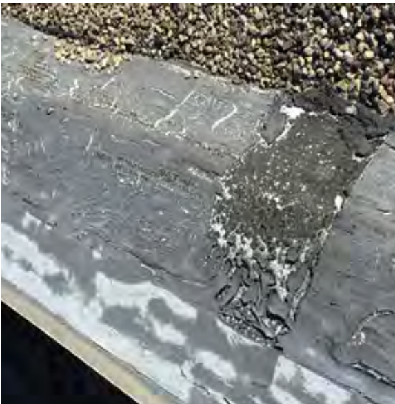
Original Edge of roof gravel stop & flashings deteriorated
