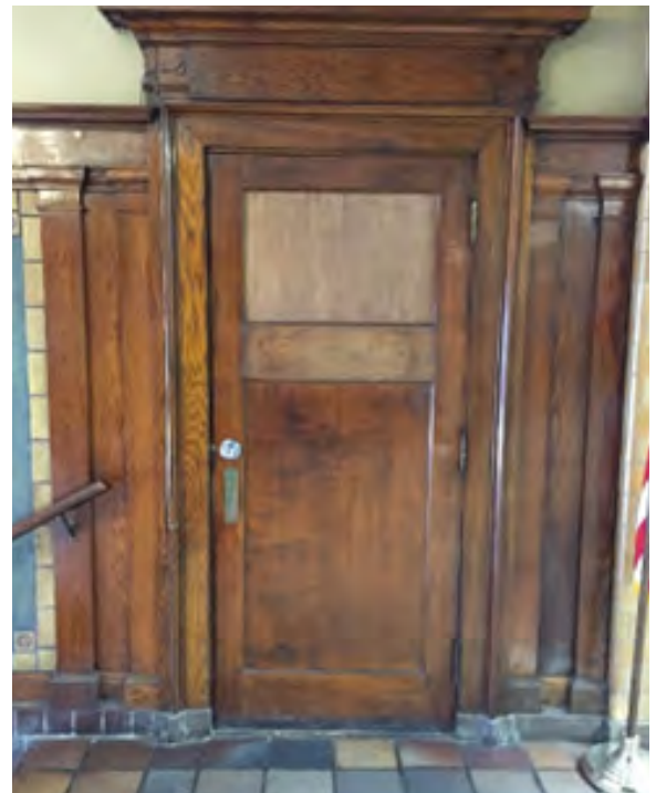
Existing interior door and trims. Hardware non-compliant.
