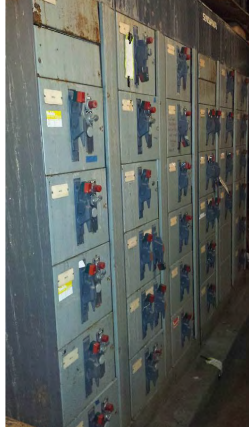
Motor Control Center
