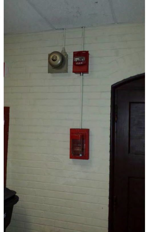
Horn Strobe and Pull Station
