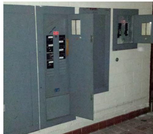
Panelboards in Kitchen
