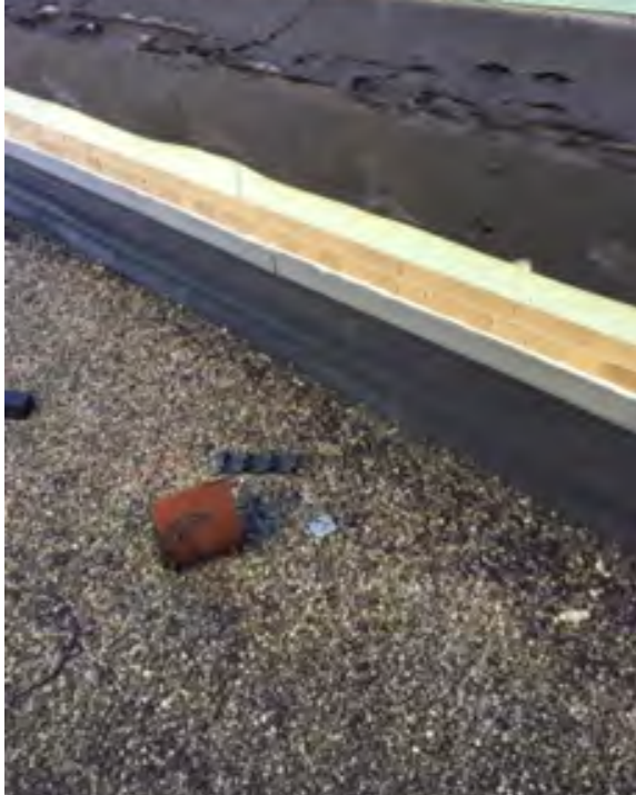
Flashings deteriorated and useless
