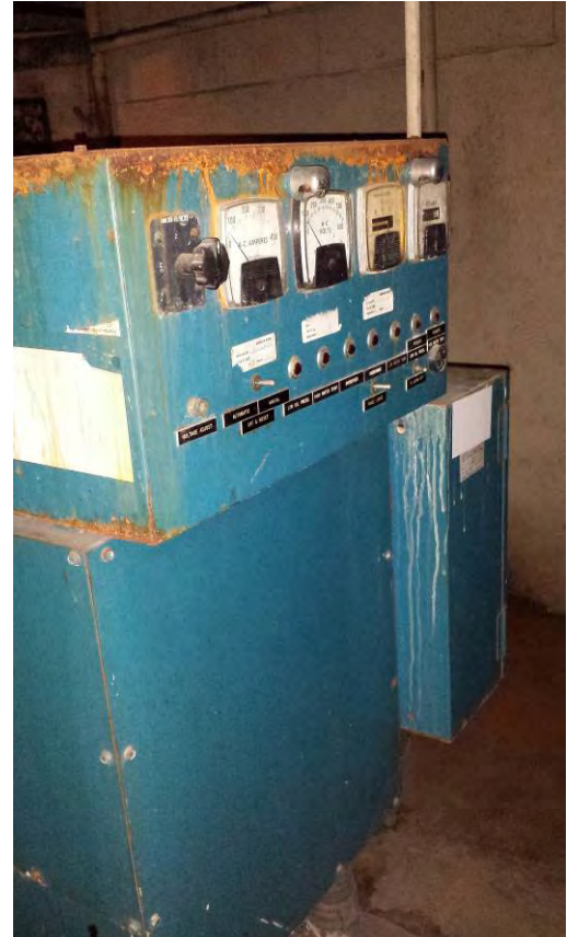
Generator Control Panel
