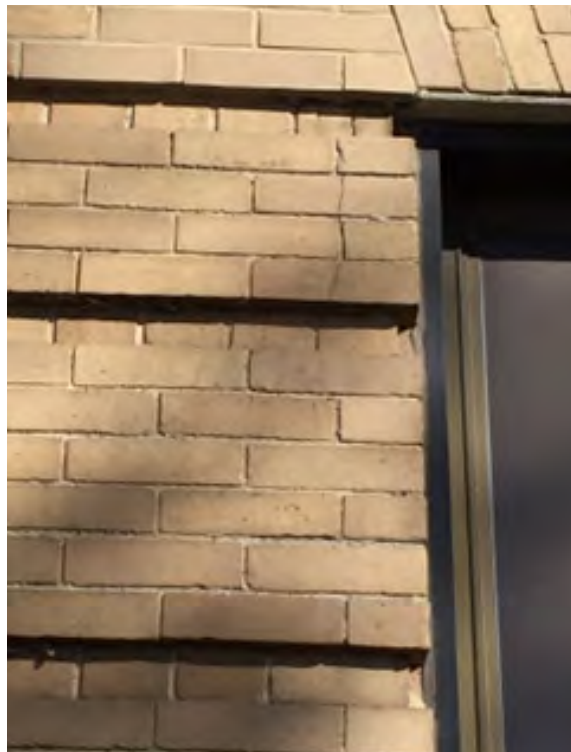
Masonry cracks and re-pointing required
