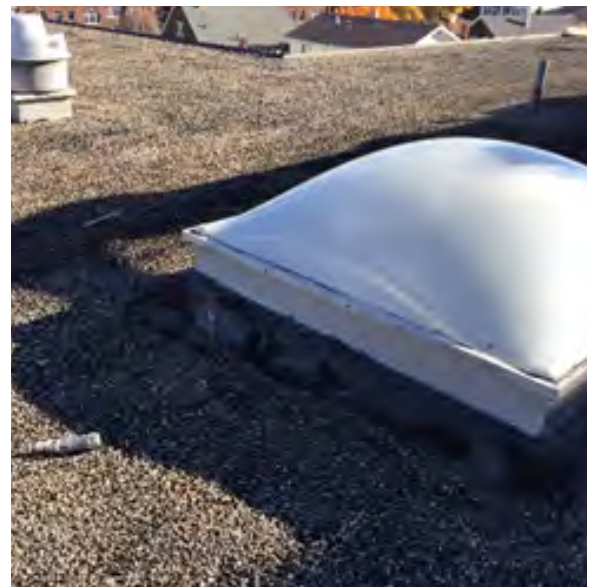
Flashings at skylights, roof fans & equipment deteriorated
