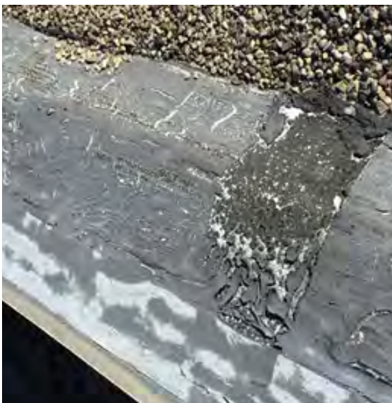
Original Edge of roof gravel stop & flashings deteriorated
