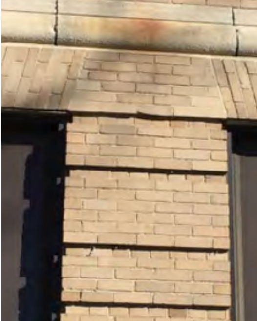
Continuous cast stone bands require repointing
