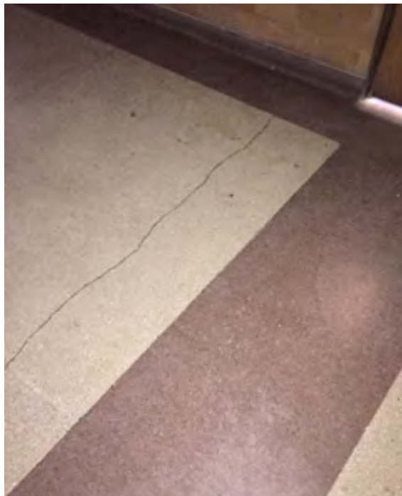
Existing terrazzo floors and cracking
