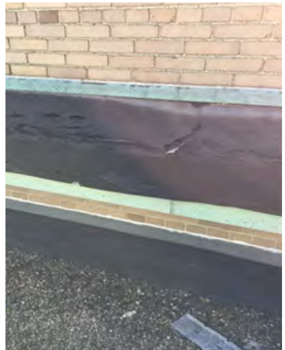
Deteriorated flashings, both copper and membrane
