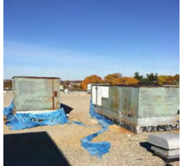
Failed and deteriorating mechanical units
