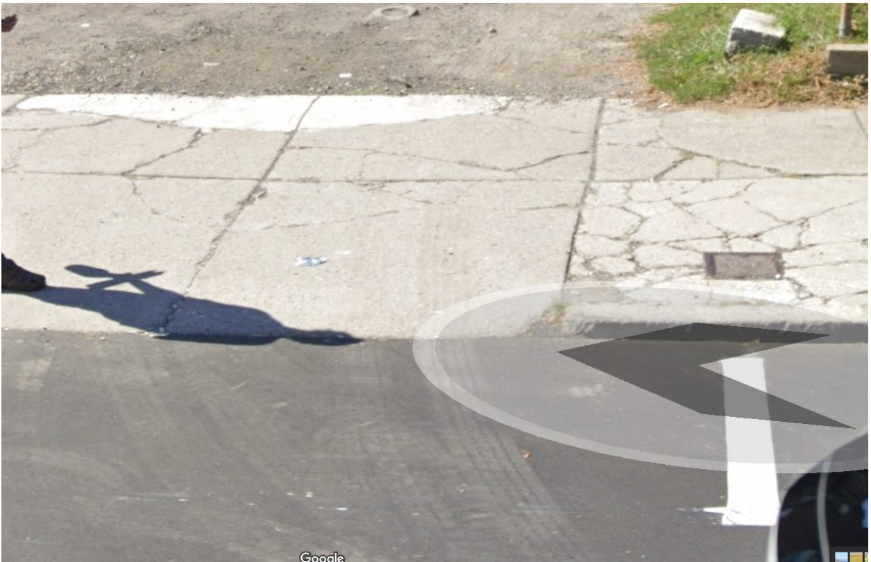
Figure 2 Cracked and broken sidewalks – typically at driveway locations
