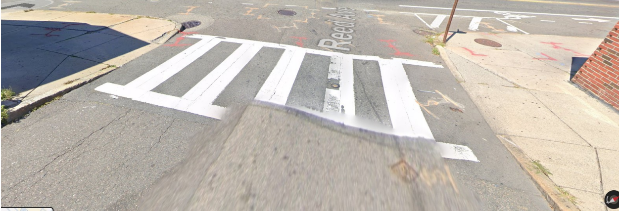
Figure 3 Non-compliant ADA ramps
