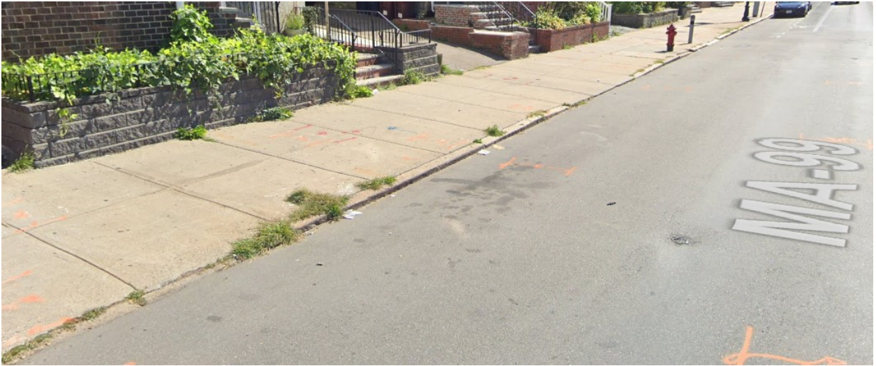
Figure 1 Sunken curb stones
