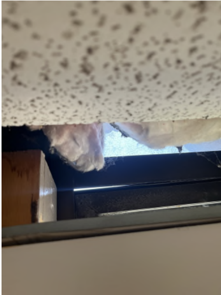
Figure 7: Window found with opening above ceiling tile grid allowing infiltration of outside air
