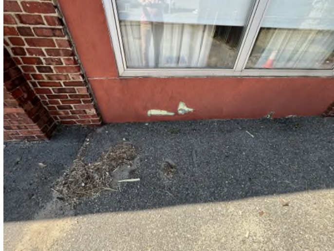
Figure 8: Damage to exterior wall of main hall exposing existing insulation
