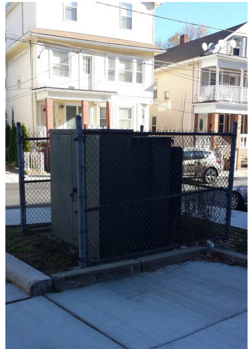
Pad Mounted Utility Transformer
