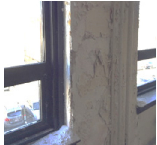
Water infiltration, wall deterioration
