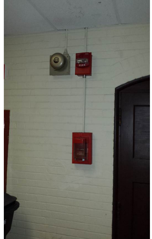
Horn Strobe and Pull Station
