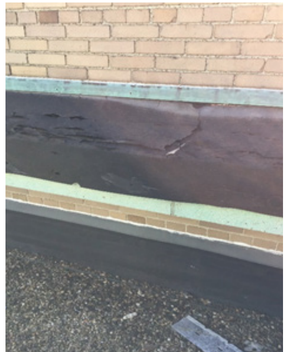
Deteriorated flashings, both copper and membrane
