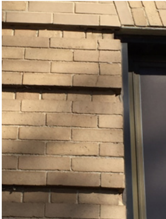
Masonry cracks and re-pointing required
