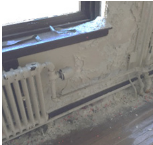
Water migration and damage to interior surfaces
