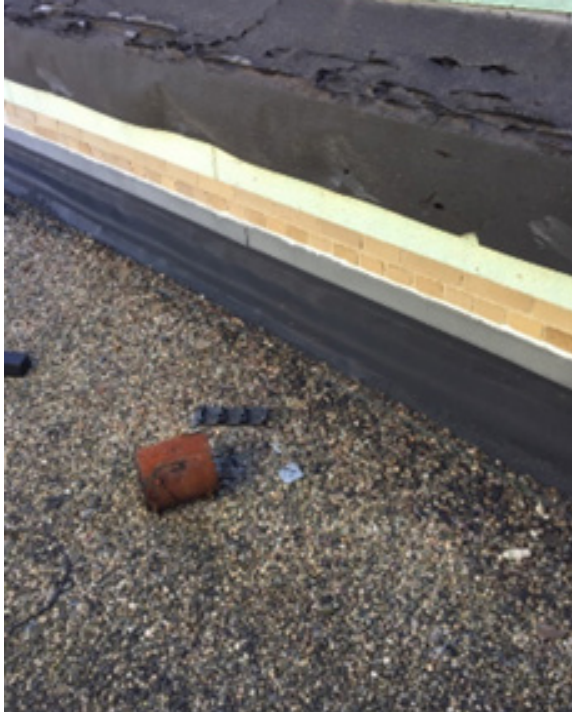
Flashings deteriorated and useless
