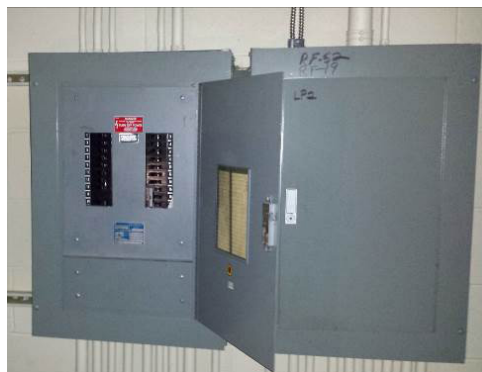
Panelboards in Electrical Room
