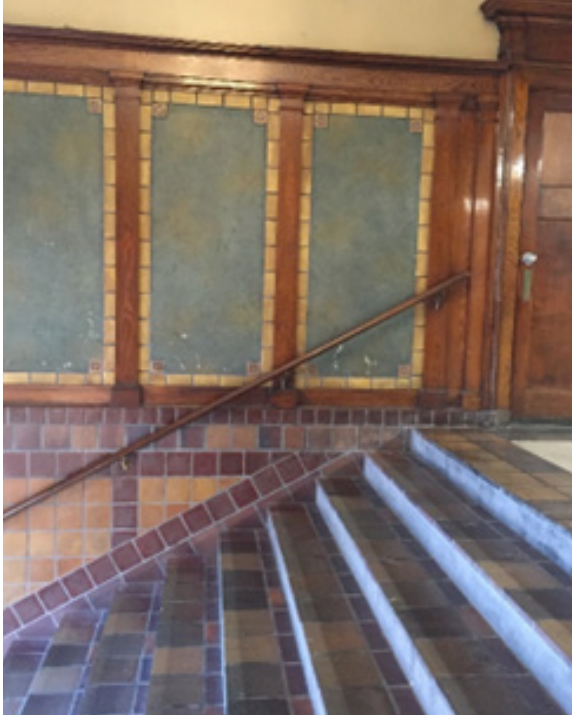
Existing interior main entry stairs non accessible
