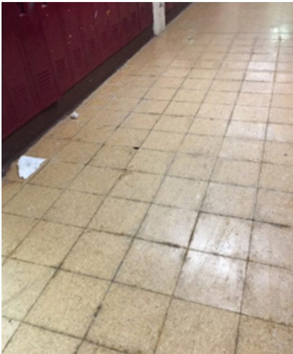
VAT & VCT worn throughout school
