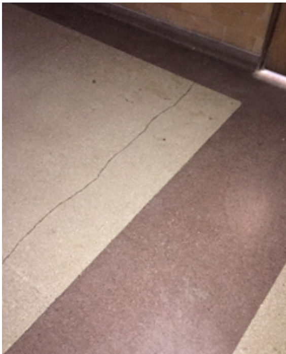
Existing terrazzo floors and cracking
