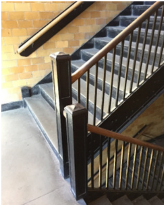
Interior stair rails and nosings non-compliant
