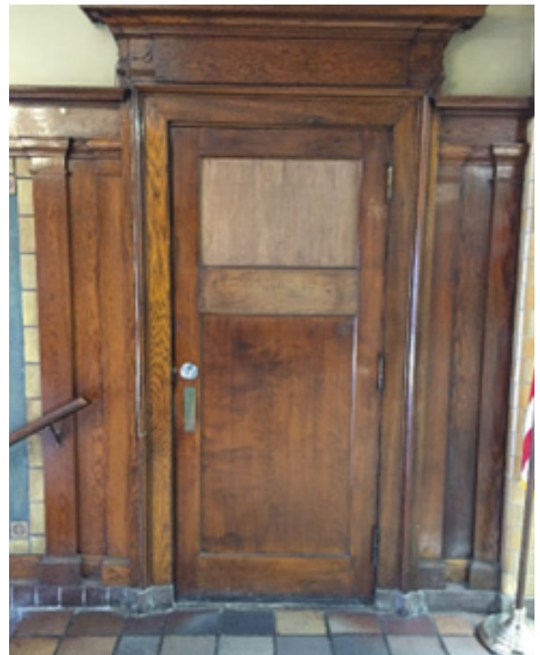
Existing interior door and trims. Hardware non-compliant.
