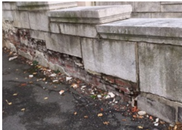
The exterior site walls at the side entrance are severely deteriorated and will require removal and replacement.
