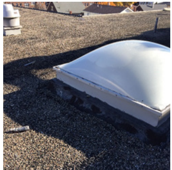
Flashings at skylights, roof fans & equipment deteriorated
