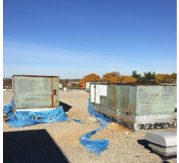
Failed and deteriorating mechanical units
