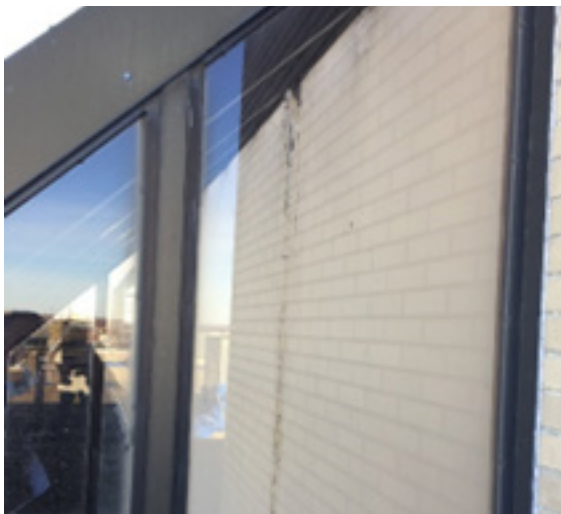
Exterior wall light leaking at inside
