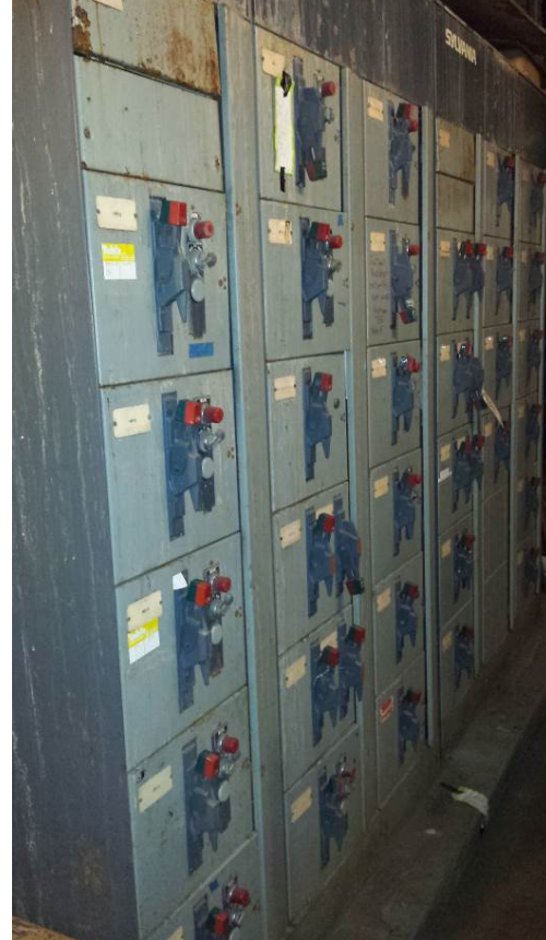
Motor Control Center
