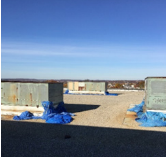
Failed and deteriorating mechanical units
