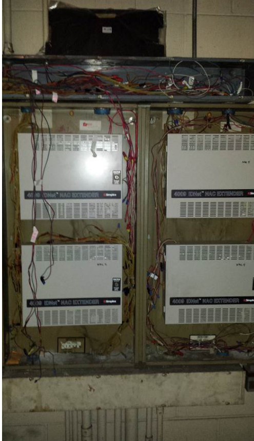
Original Control Panel with new Equipment
