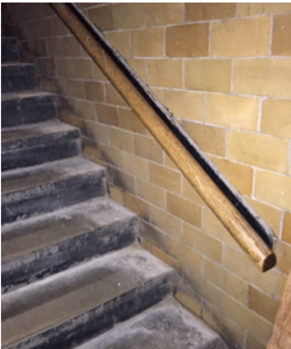
Non-Compliant rails and stair tread nosings
