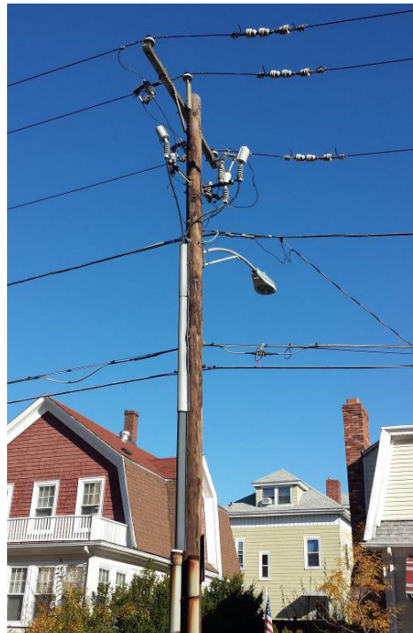
Utility Pole with Incoming Utility Primary Lines
