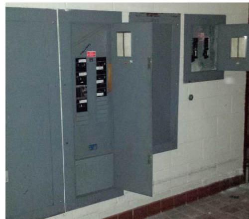
Panelboards in Kitchen
