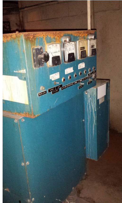
Generator Control Panel
