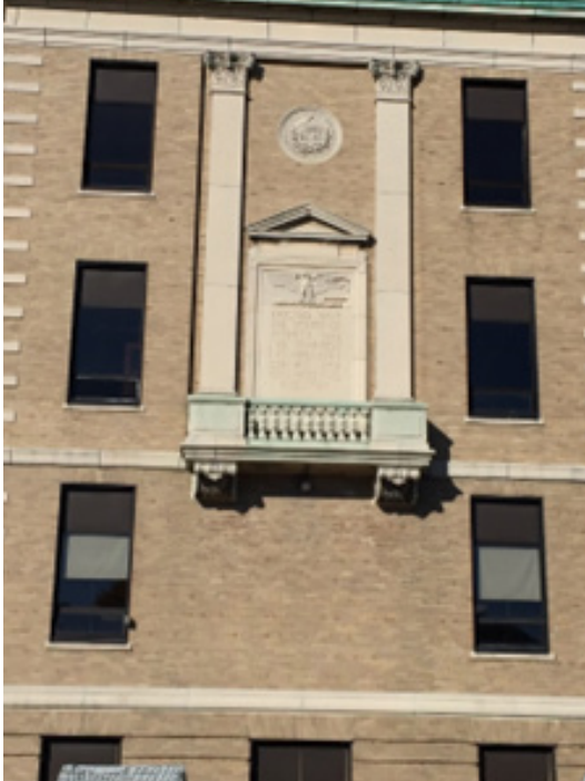
Copper cornice flashings deteriorating
