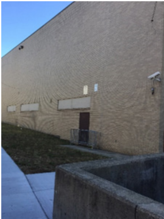
1970's addition facing Linden Street Boarded window openings
