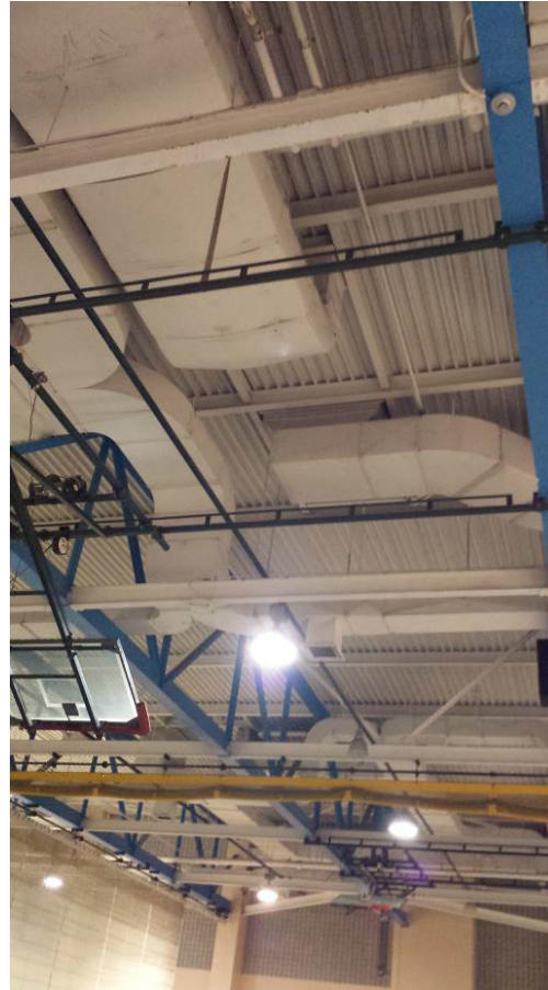
High Bay HPS in Gymnasium
