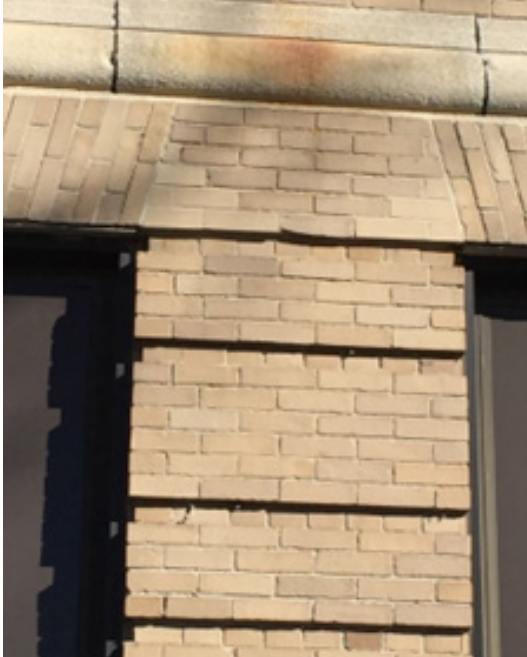
Continuous cast stone bands require repointing
