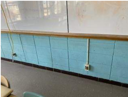
Typical Classroom Telecomm. Devices
