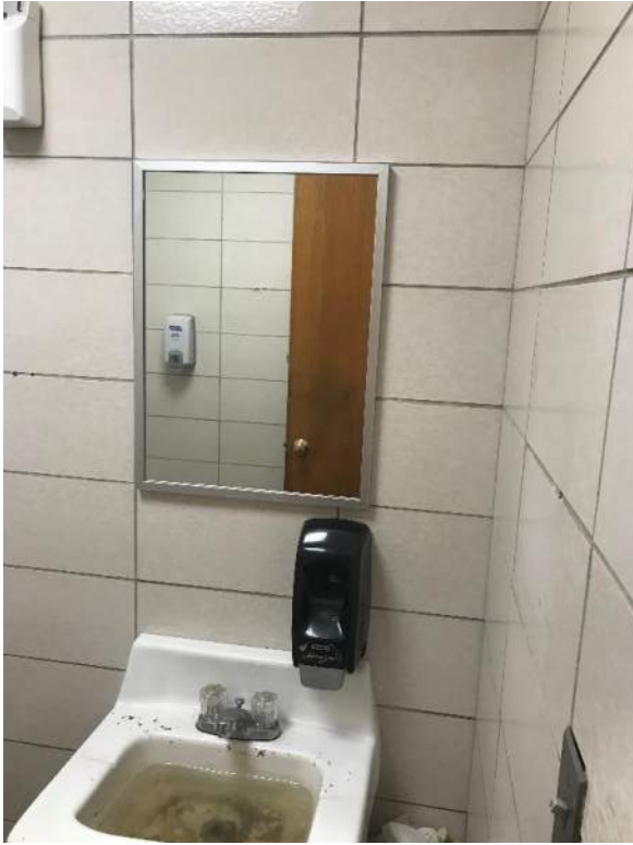
Sink faucets, height, height of mirror and accessories not Handicap accessible
