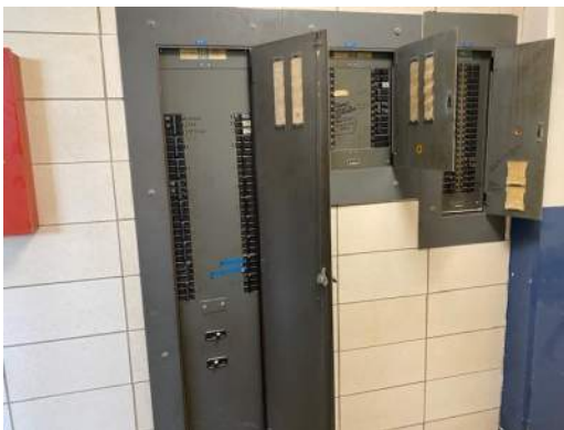
Typical Older Style Sub-Panels
