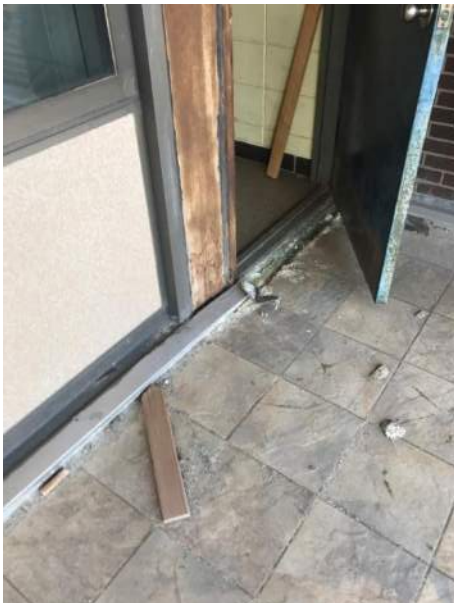
Door sill deteriorating at exterior covered walk
