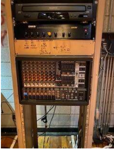
Auditorium Sound System
