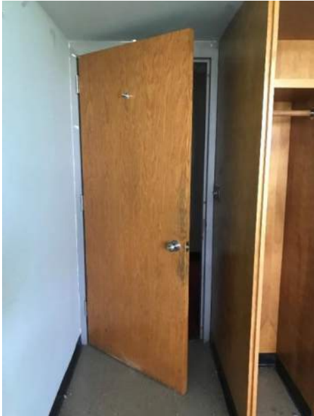
Door to convent room, no handicap hardware, not accessible on pull side
