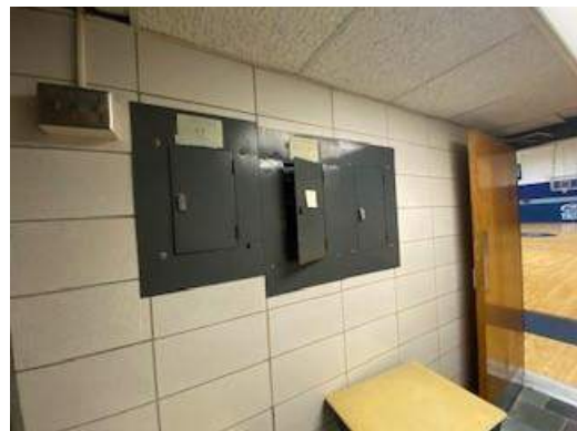
Typical Corridor Flush Sub-Panels
