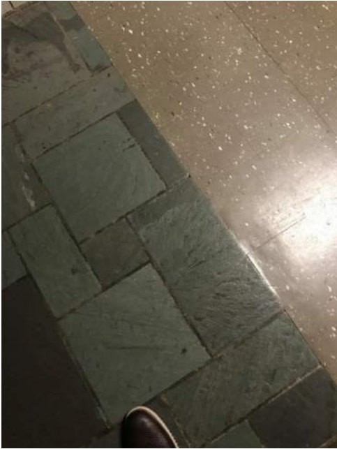
Random bluestone pavers and VAT abut, no transition strip
