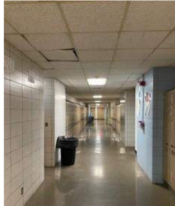
Typical Corridor Lighting
