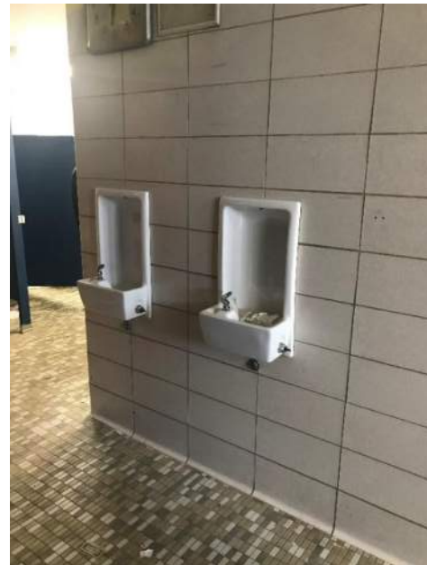
Existing drinking fountains to be replaced
