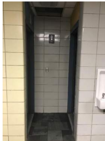
Stack bond structural glazed block Entrance to toilets not handicap accessible
