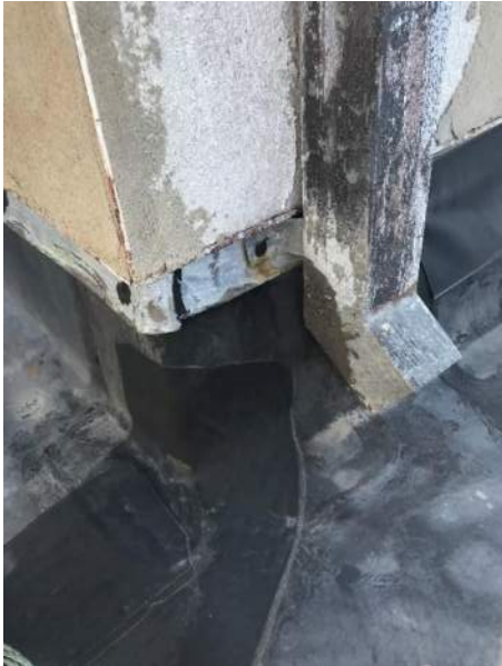
Downspout deteriorating, plaster spalling
