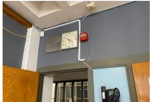
Typical Classroom Sound Speakers, Clock, & Telephone
