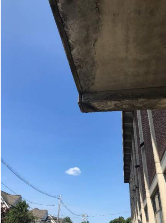
Concrete soffit spalling
