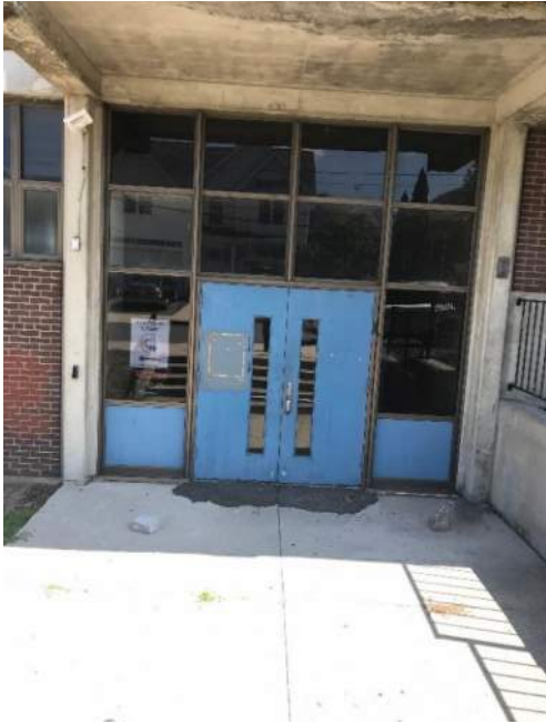
Existing metal doors and frames in poor condition
