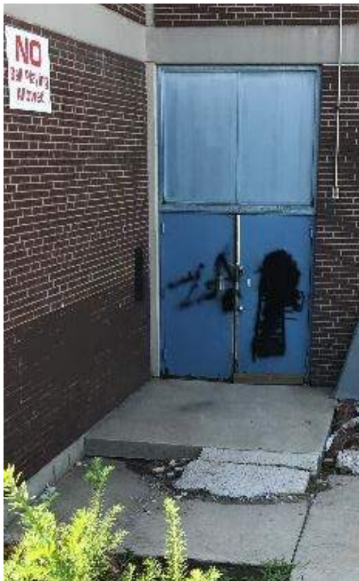
Doors and frame in poor condition/no accessibility
