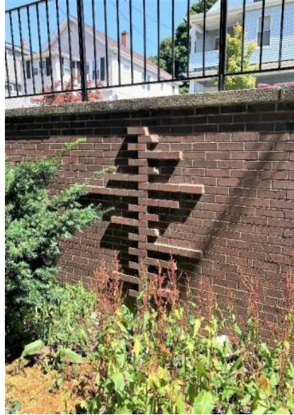
View of exterior masonry site retaining wall at north side of site that shows deteriorated / spalled brick.
