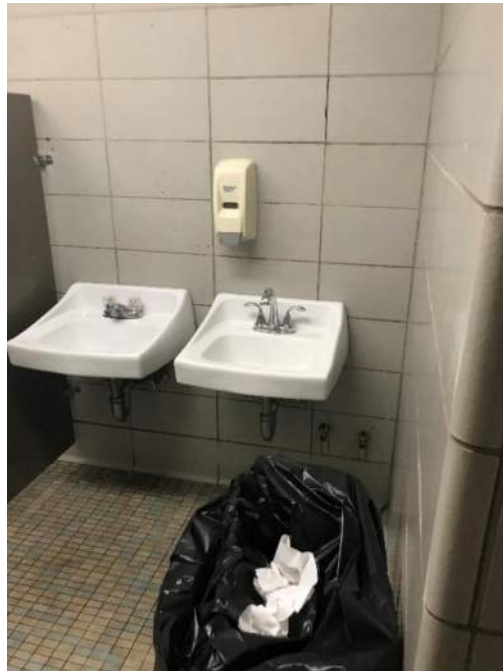
Sinks, no mirrors, and soap dispenser Drain pipes below handicap sink should have protective coverings
