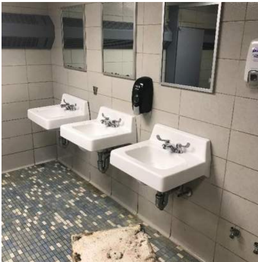
Sinks, mirrors, and soap dispenser Drain pipes below handicap sink should have protective coverings. No handicap accessibility
