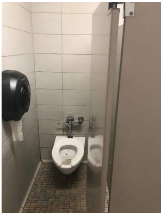
Toilet stall, typical not handicap accessible No grab bars, accessory heights not accessible
