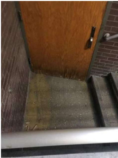
Door swing and egress not acceptable
