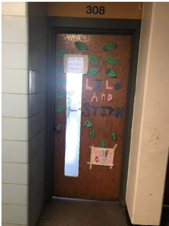
Pocketed door classroom entry, not handicap accessible
