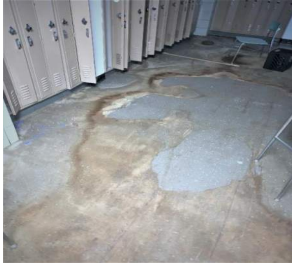
Signs of water staining on first floor slab-on-grade, which is evident of a previous leak.
