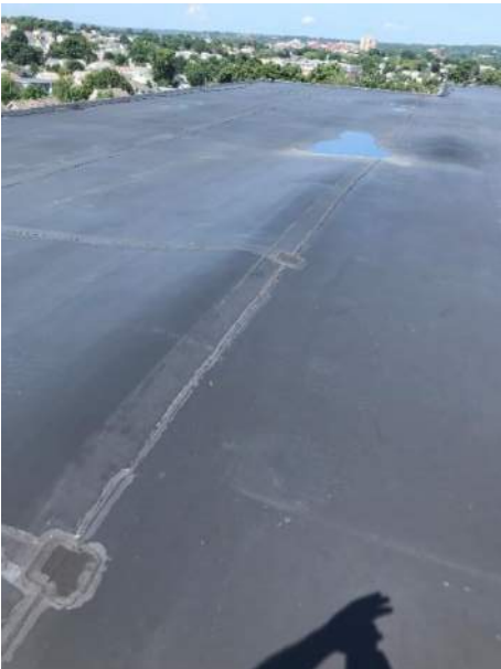
Insulation and membrane ballooning
