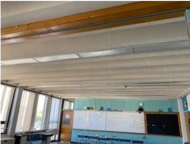
Typical Classroom Lighting
