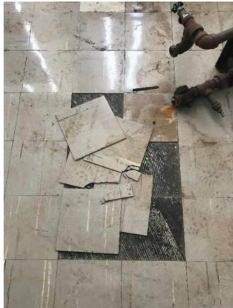
Water damaged VAT flooring
