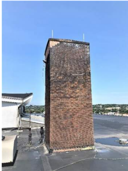
View of brick chimney that will require structural repairs / repointing.
