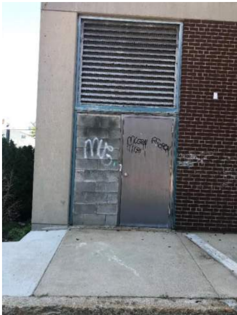
Metal door and frame and louver in poor condition, concrete pad exit
