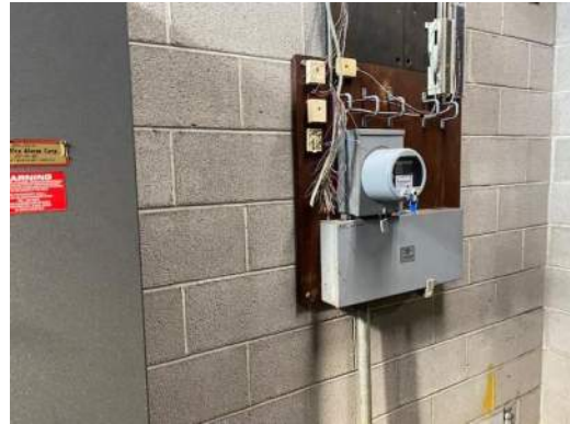
Utility Company Meter
