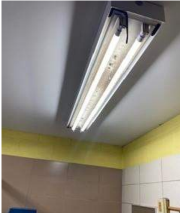
Typical Retrofitted LED Light Fixture
