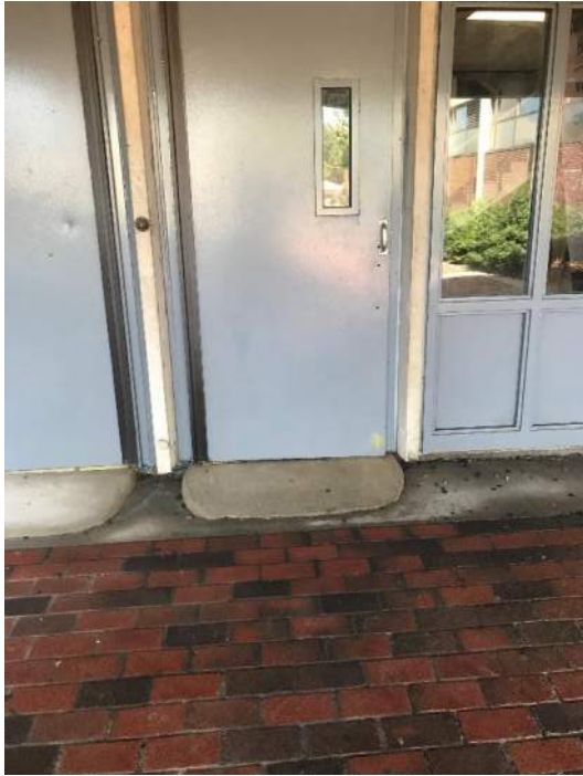
Feathered concrete sills at entry doors
