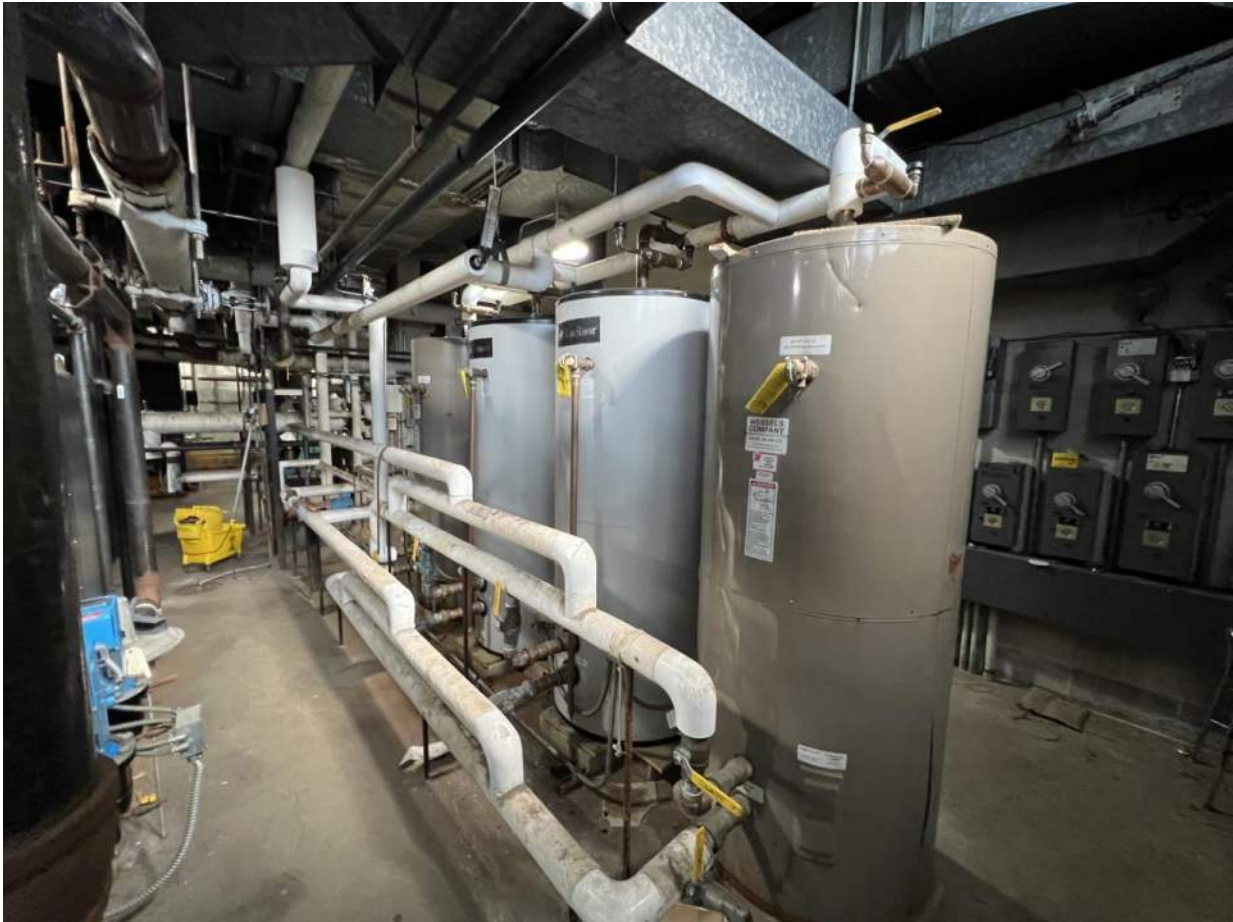
Domestic Hot Water Tanks
