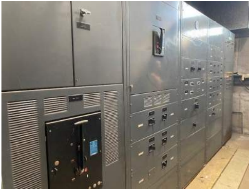
Main 2500Amp Distribution Board
