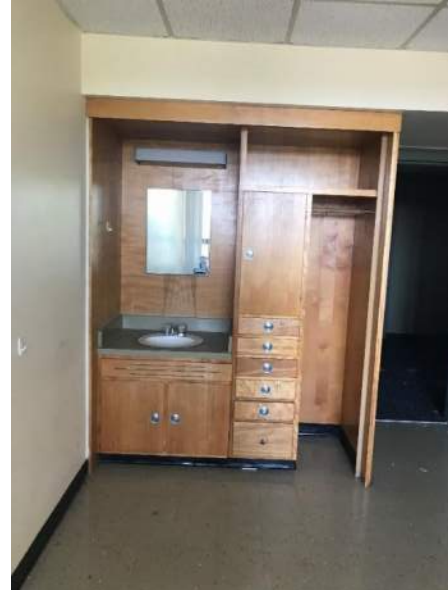
Sink to be ADA if it is to remain
