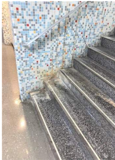
Water damage / mold along interior stair wall.
