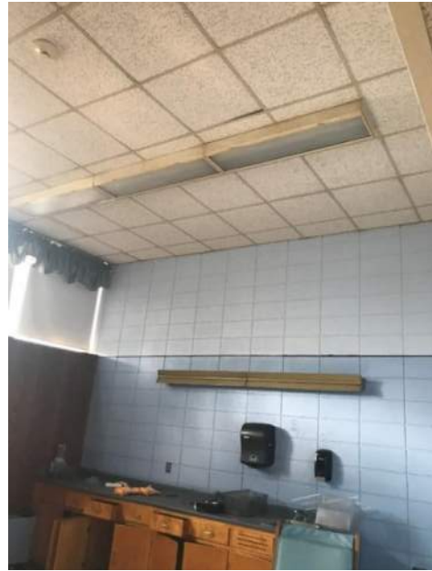
2x2 Acoustic tile and metal grid 1 X 4 Surface mounted lights
