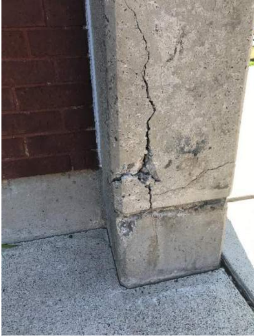
Exterior vertical concrete column cracked at base
