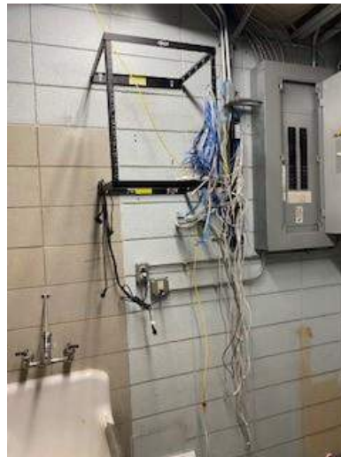
Main IT Room
