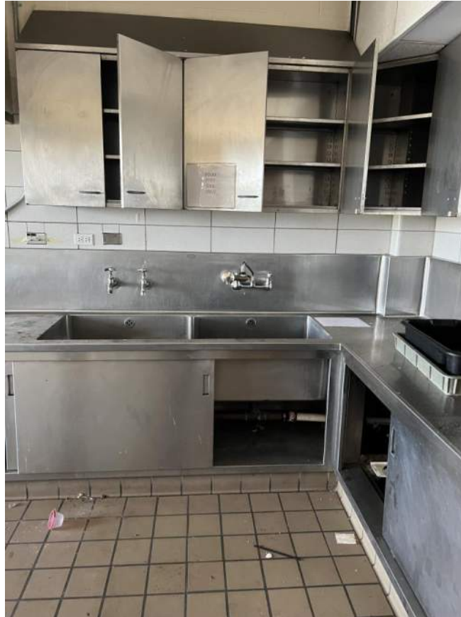
Prep. Sink with PVC repair (not indirectly wasted)
