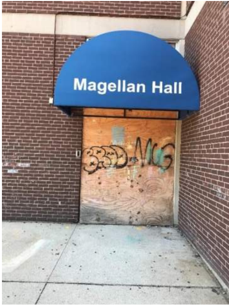
Existing entry boarded
