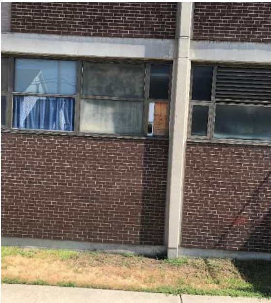
Existing windows original to building, sealants To be replaced
