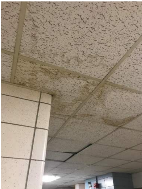
Water damaged tiles
