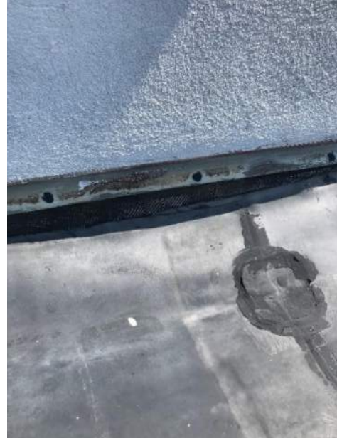
Termination bar/membrane failing
