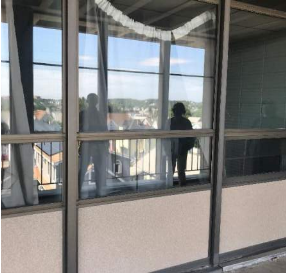
Typical single pane metal windows and panel base At covered patio area
