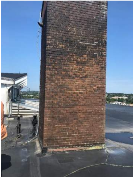
Boiler chimney, requires repointing and Structural repairs
