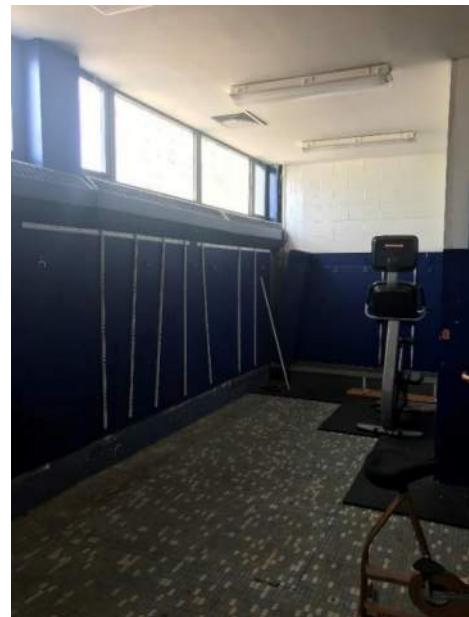
Plaster ceiling w/ 1x surface mount lights
