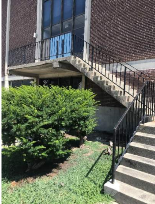
Exterior concrete egress/entry stair not accessible
