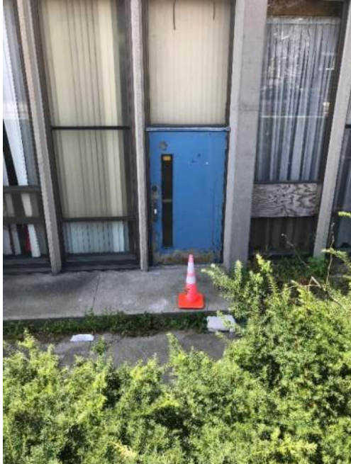
Metal door and frame in poor condition, concrete pad exit No accessibility.
