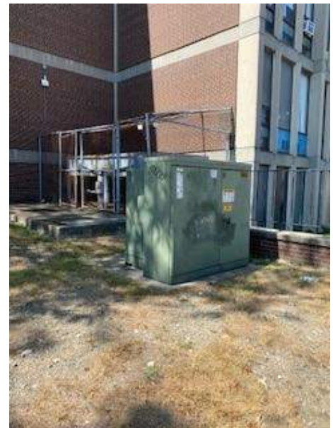
Utility Company Pad-mount Transformer
