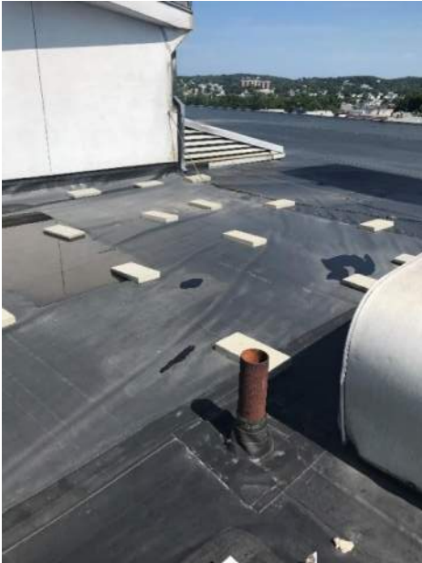
EPDM temporary patch
