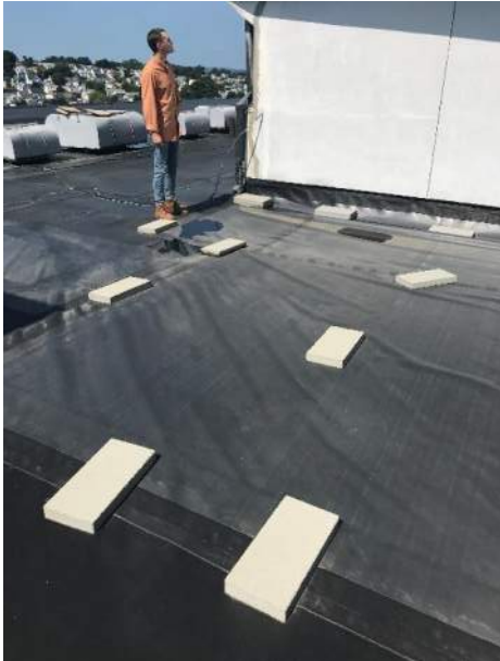
EPDM membrane patch held down with Concrete blocks
