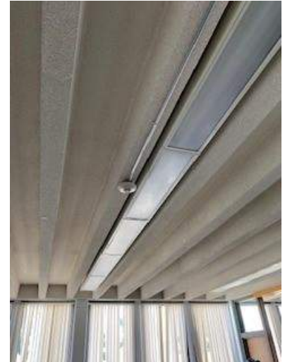
Typical Classroom Smoke Detector
