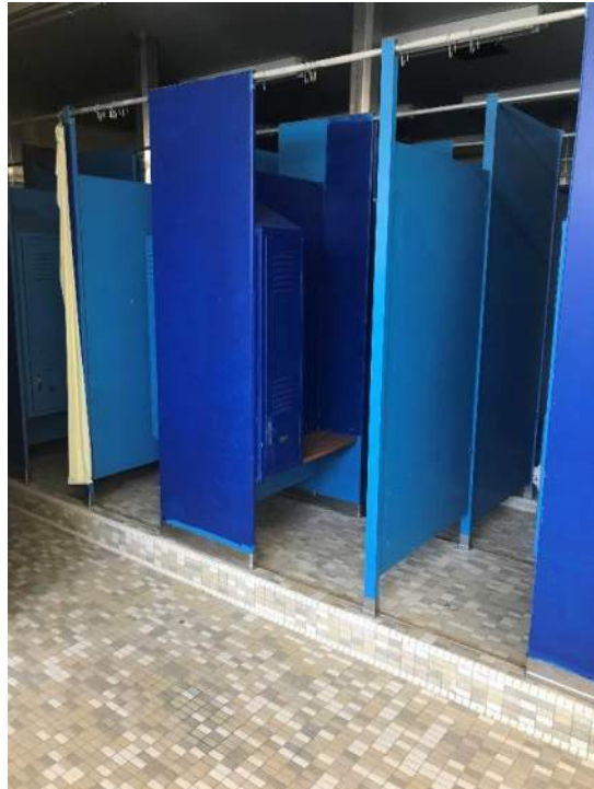
Existing girls dressing/shower areas. Not handicap accessible
