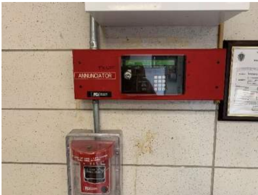
Fire Alarm Annunciator & Typical Pull Station w/ Plastic Guard
