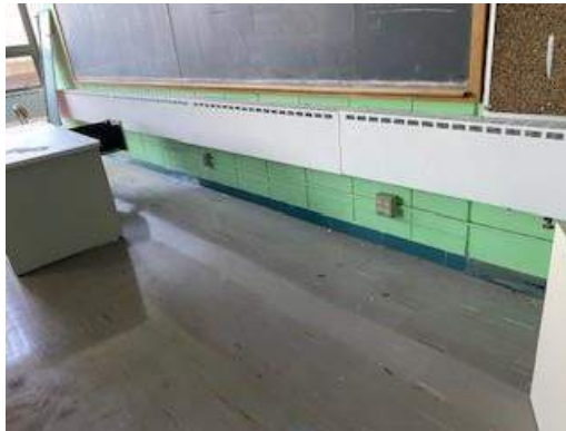
Figure 1 Typical wall receptacle & Surface raceway
