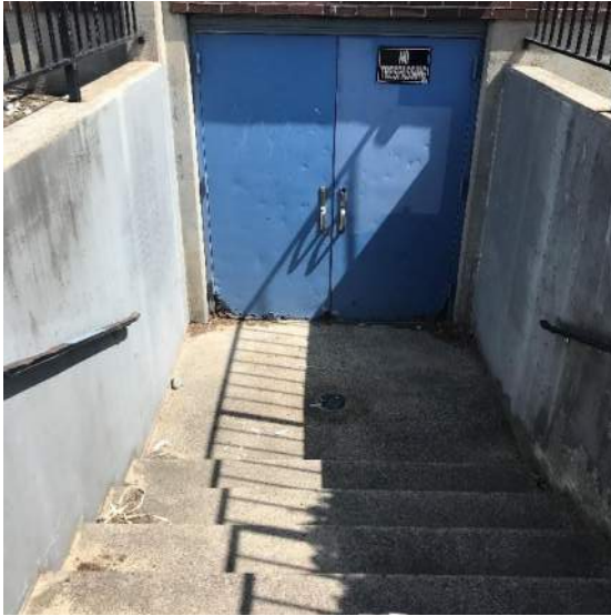
Doors at base of exterior stair rusting and dented
