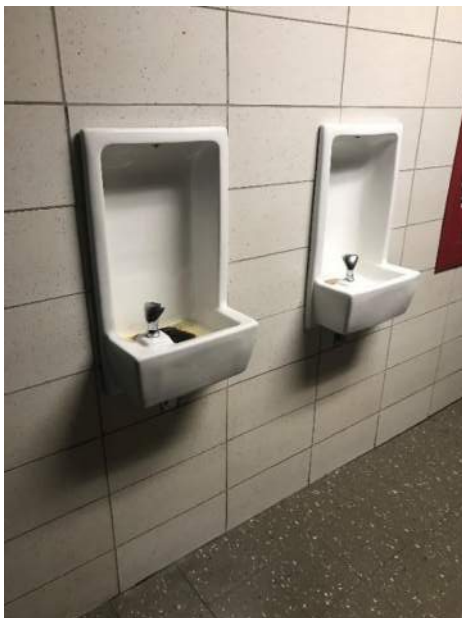
Existing drinking fountains throughout should be replaced with new and handicap accessible units
