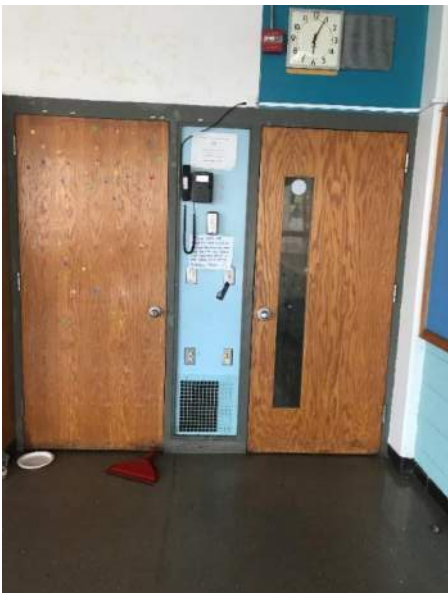
Typical classroom and storage door No handicap hardware
