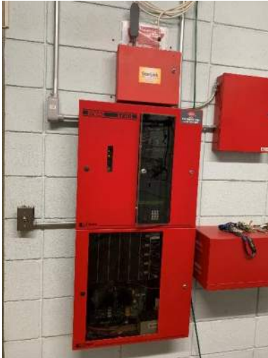
Main Fire Alarm Control Panel
