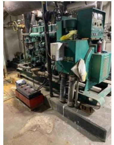
Manual 125-KW Natural Gas Generator
