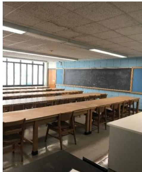
Typical classroom tiles with surface mounted fixtures. Water damage
