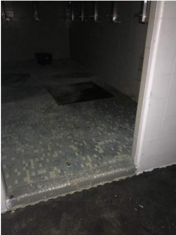
Shower stall curb/ not handicap accessible
