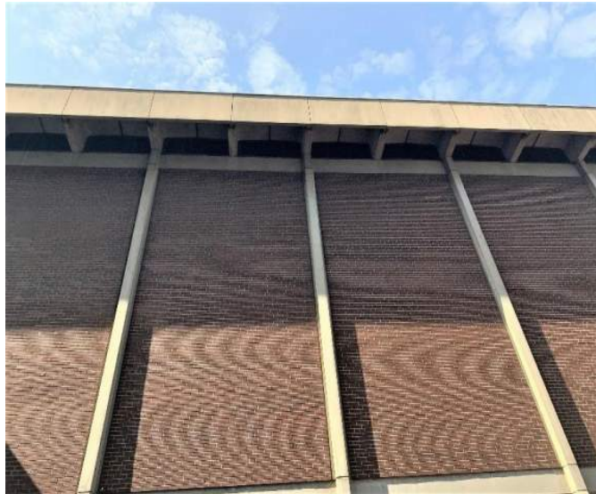
View of exterior masonry wall adjacent to gymnasium in Part A that shows cantilevered precast prestressed concrete single-tees at the roof level.
