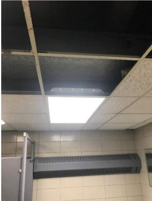
2 x 4 tiles and grid in toilets. Tiles missing
