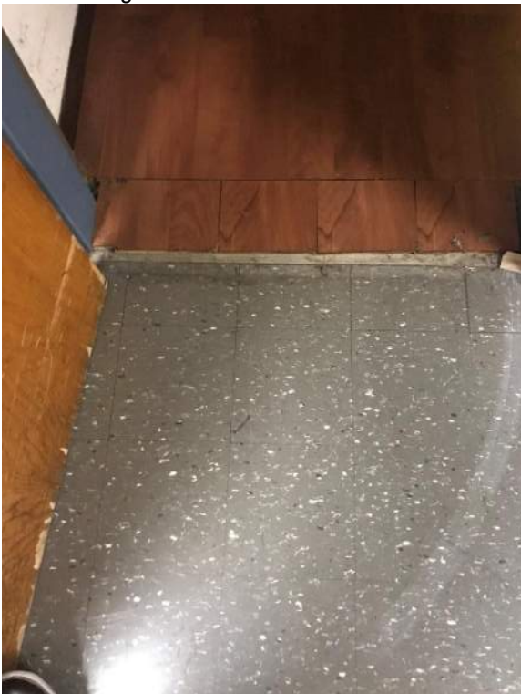
VAT flooring abutting newer composite wood floor system
