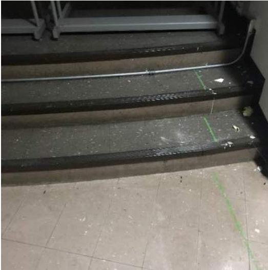
VAT at stair landings and stair treads, treads with nosing
