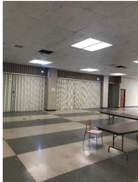
2 x 4 tile appears to have been painted
