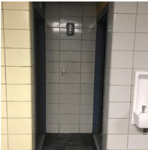
Entry to toilet rooms / Not a handicap accessible entry
