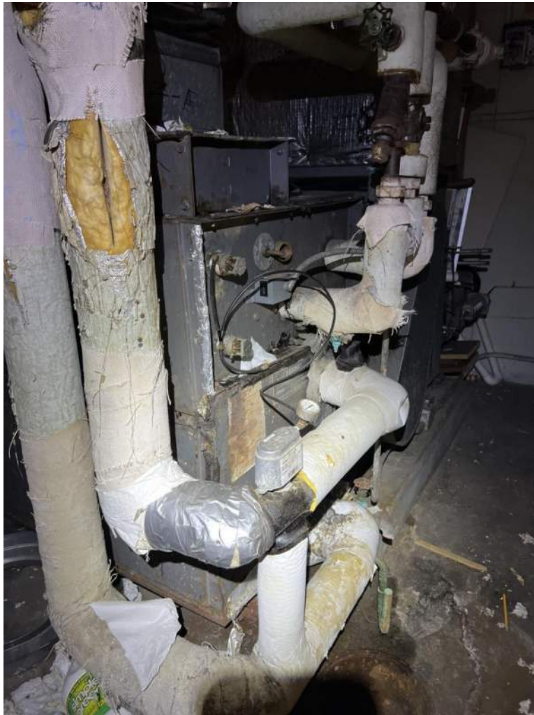
Air Handling Unit (Cooling and Heating)
