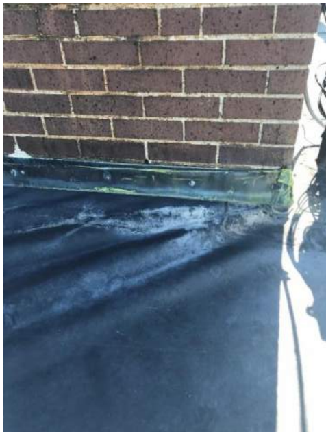
Roofing buckling at wall termination
