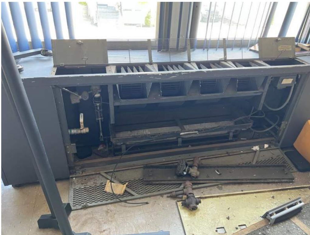
Unit Vent – Draw Thru Style (coil in process of being replaced)
