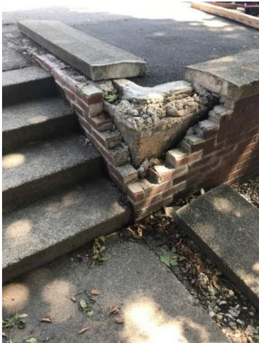
Exterior site stair/wall needs repair
