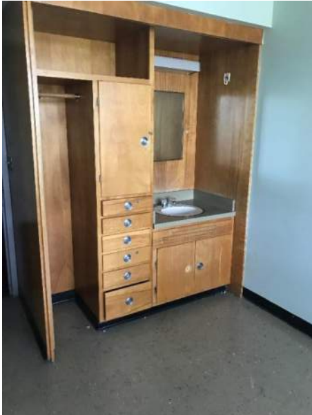
Dressing unit and sink in the convent area Sink should comply w/ ADA if it is to remain
