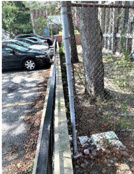
View of site retaining wall that has deteriorated and appears bowed, which will require structural repairs.
