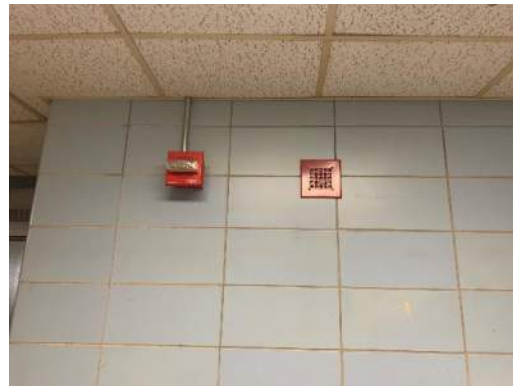
Typical Horn/Strobe & Voice Evacuation Devices
