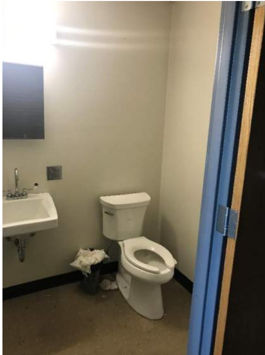
Single user toilet not handicap accessible
