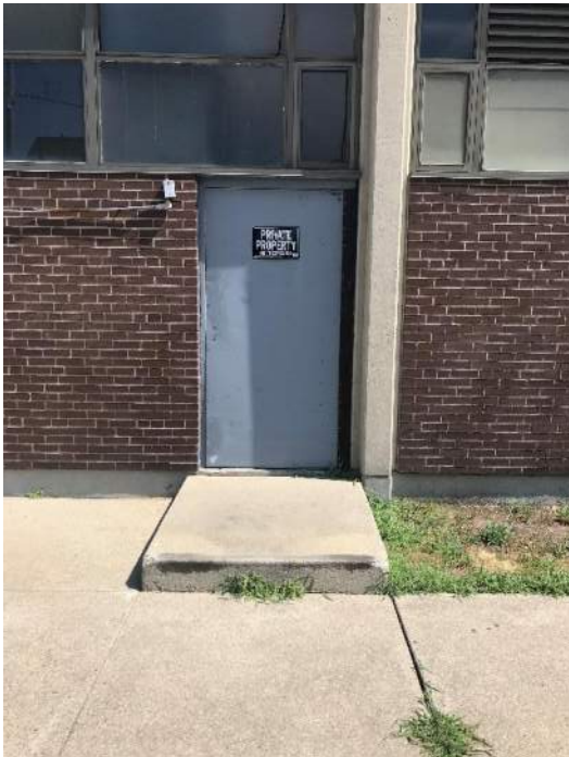
Metal egress door, windows and frames in poor condition
