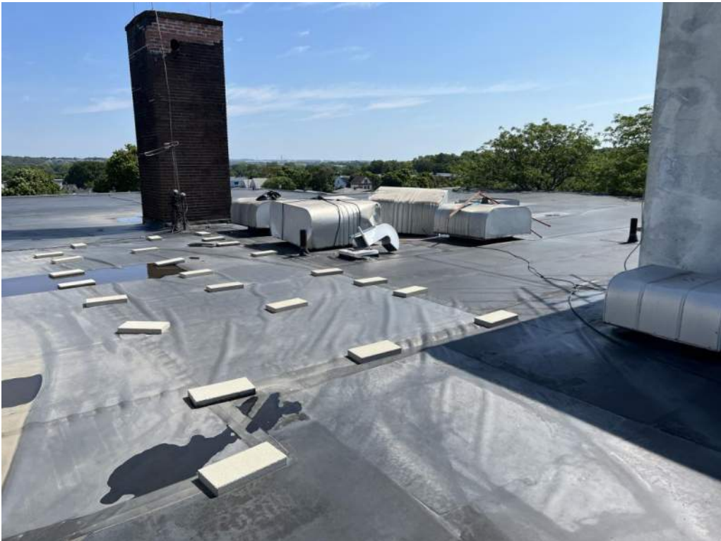
Damaged Roof Fan, Fan off Curb and Gooseneck Duct Broken
