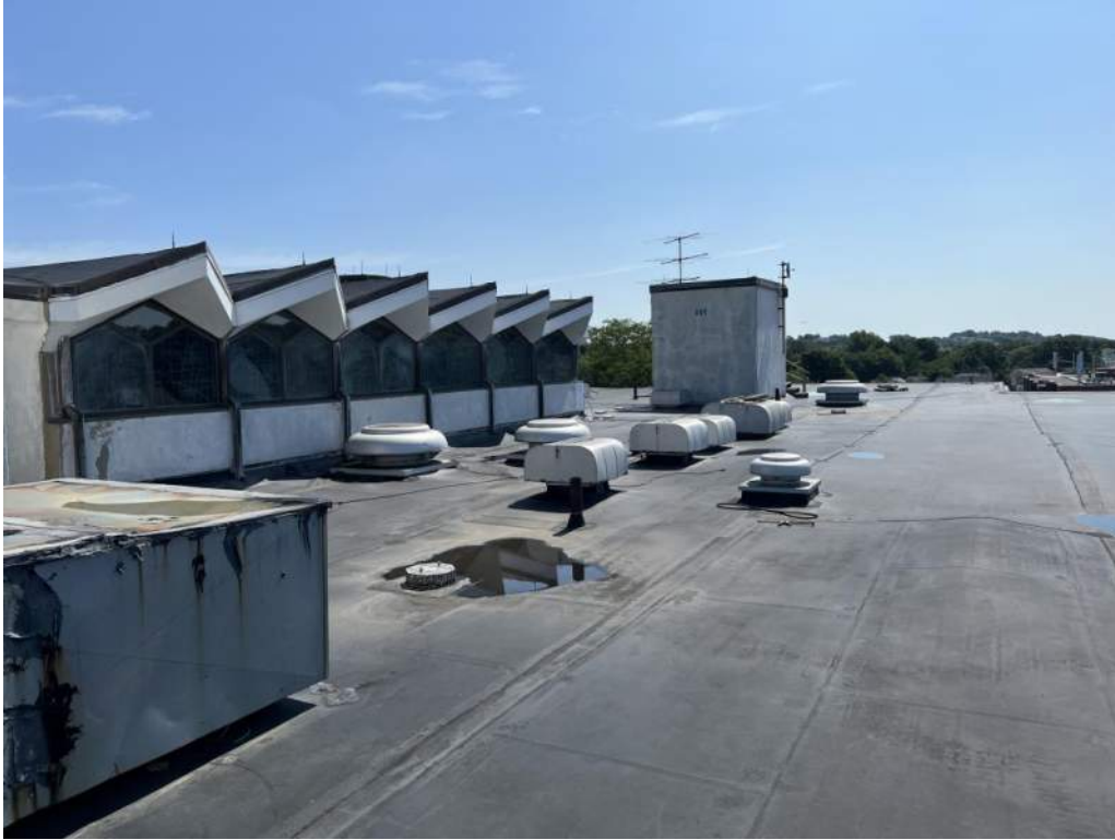
Roof Fans and Intakes
