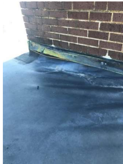
Roofing buckling at wall termination and metal broken from wall
