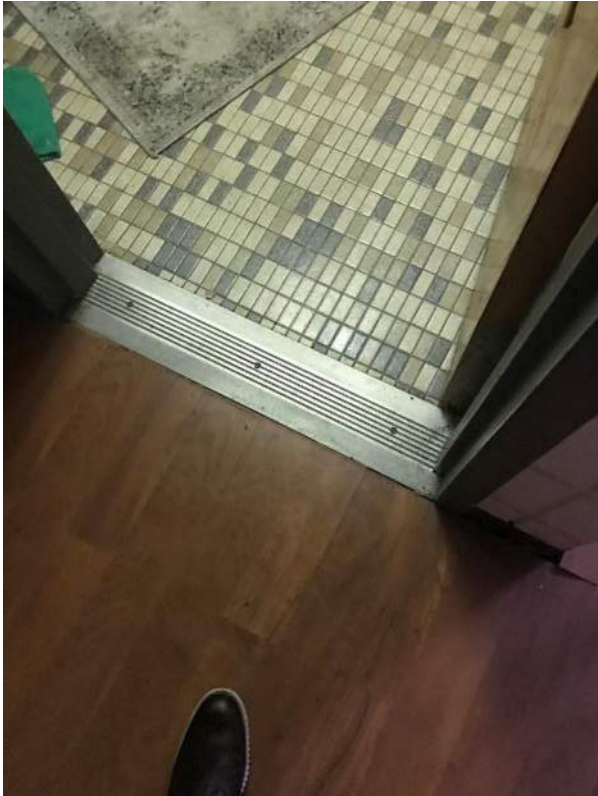
Composite flooring, aluminum sill & ceramic tile toilet floor
