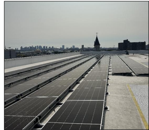
Solar array atop City Hall
